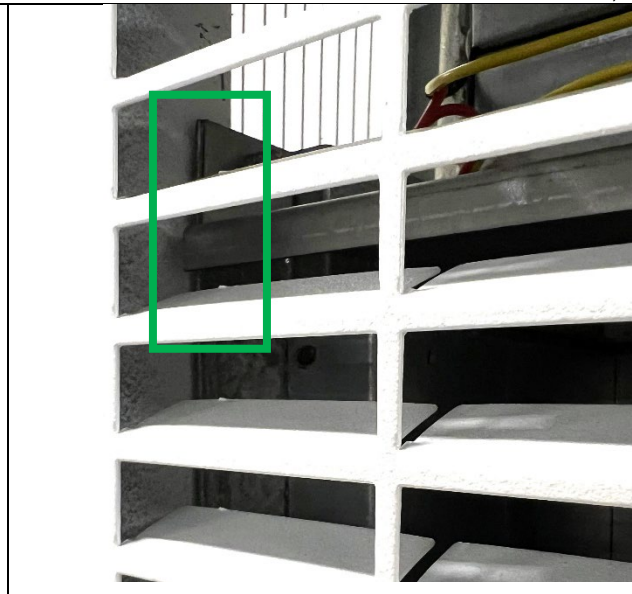
Good install: No gap
